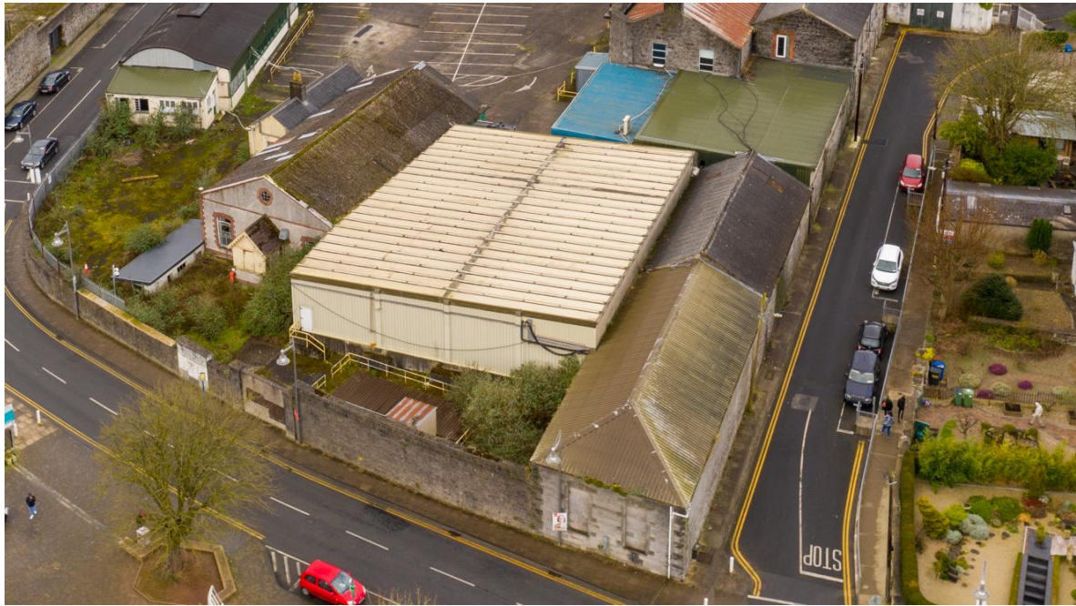
Figure 26 - Linen Store from above. Modern cold store abutting and the alterations to the northern cells in the form of a raised and replaced roof.
